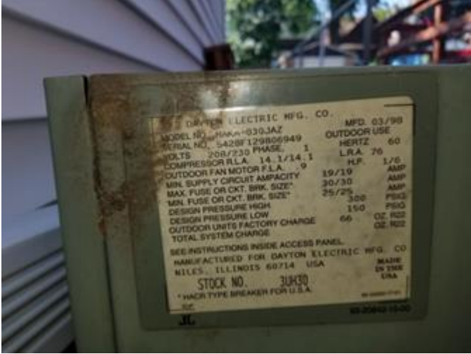
HVAC - Cooling System
